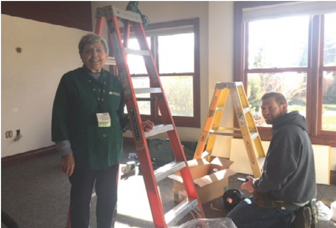
Carol DeBauche, volunteer, joined Chris Zimmerman, electrician, during the renovation of a patient room.
